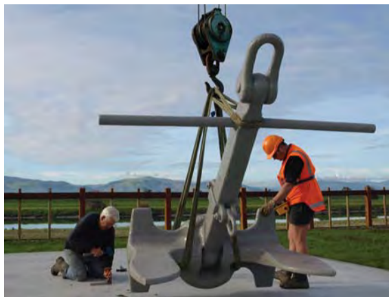
Above: Project manager Lawrie Smith makes some final adjustments on the anchor's new site
