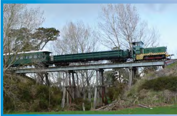
Above: The rail bridge over the Waitete Stream is a vital link on the Waihi to Waikino line.
