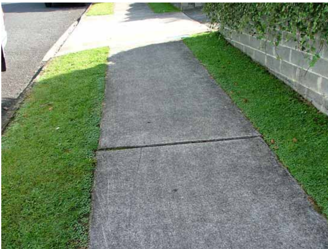
Photos 1&2 Cracking in Haszard Street with an unusual north (pit wall) side up and small right lateral component, suggestive of large “block” movement on a through-going rock mass defect.
