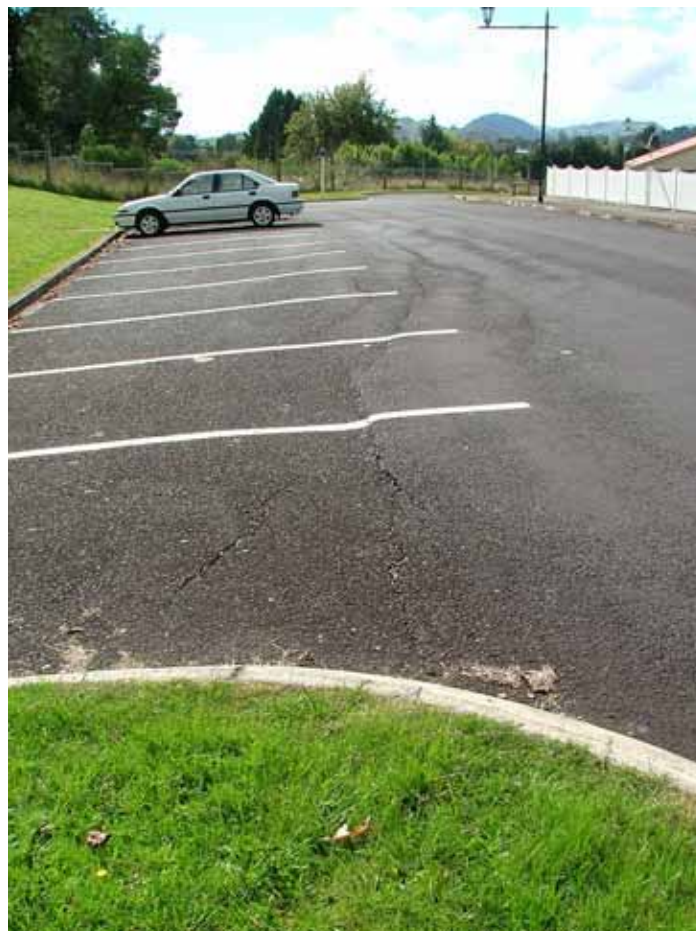
Photos 3&4 Cracking in Seddon Street appears to be extensional but also has a small right lateral component of movement in the pavement above.
