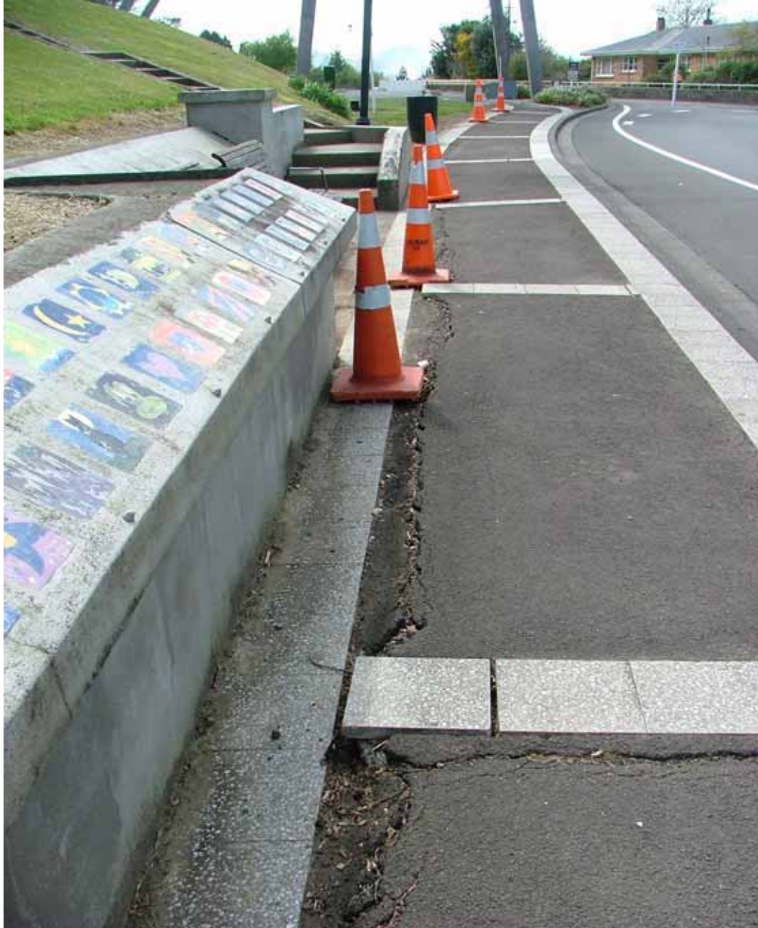
Photo 5. Ground cracking due to lateral northward movement and subsidence, evident along the base of the Millennium Wall in Seddon Street, Sept 2008.
