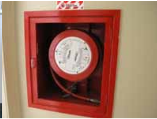
Rear Toilets Hose Reel
