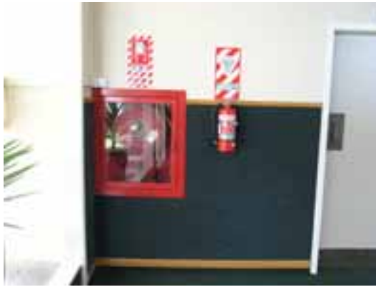
Foyer Fire Extinguisher and Hose Reel
