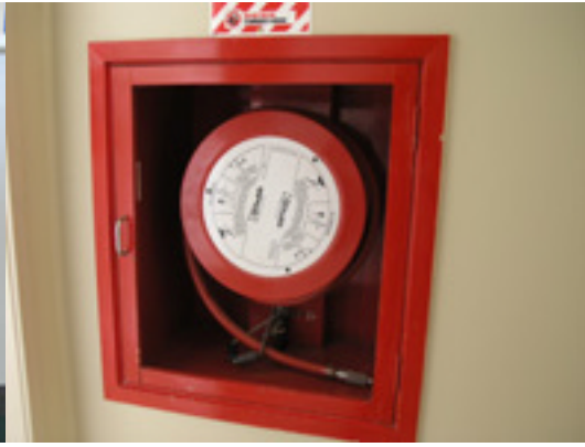
Rear Toilets Hose Reel
