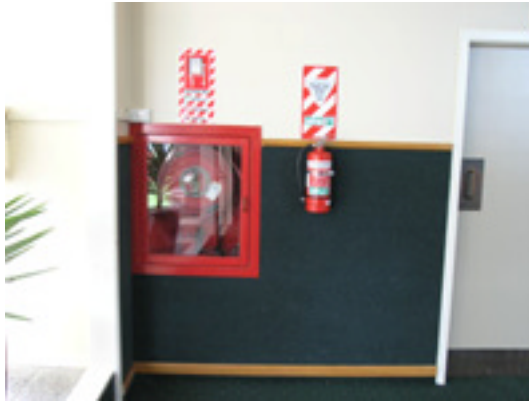
Foyer Fire Extinguisher and Hose Reel
