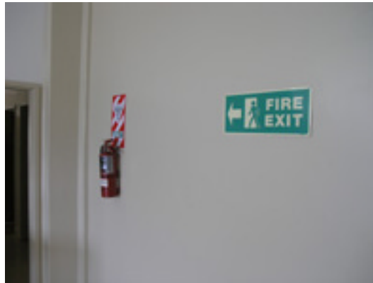
Kitchen Fire Extinguisher
