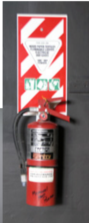
Main Stage Fire Extinguisher
