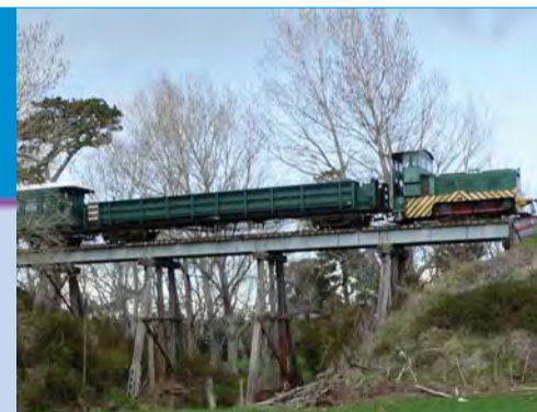
Above: The rail bridge over the Waitete Stream is a vital link on the Waihi to Waikino line.
