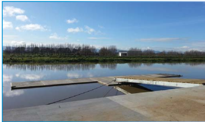
Ready to launch: The finished pontoon in the calm waters of the Piako River. Photo courtesy of Mike Speedy
