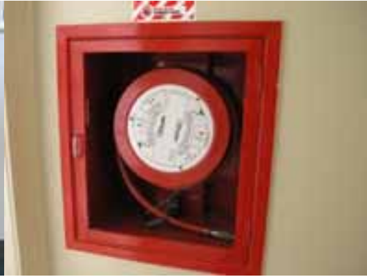
Rear Toilets Hose Reel
