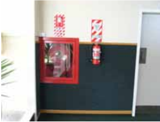
Foyer Fire Extinguisher and Hose Reel
