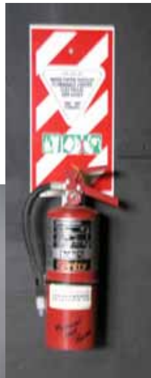
Main Stage Fire Extinguisher
