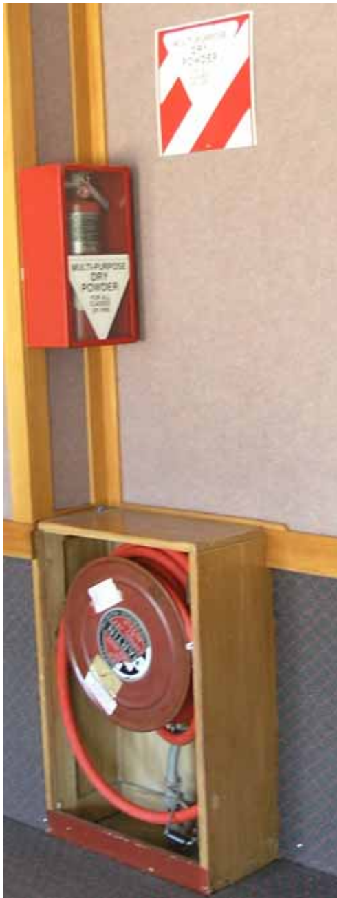
Foyer Fire Extinguisher and Hose Reel
