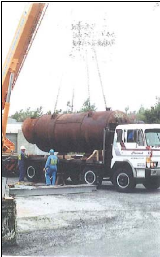
Boiler tank on to transport.
