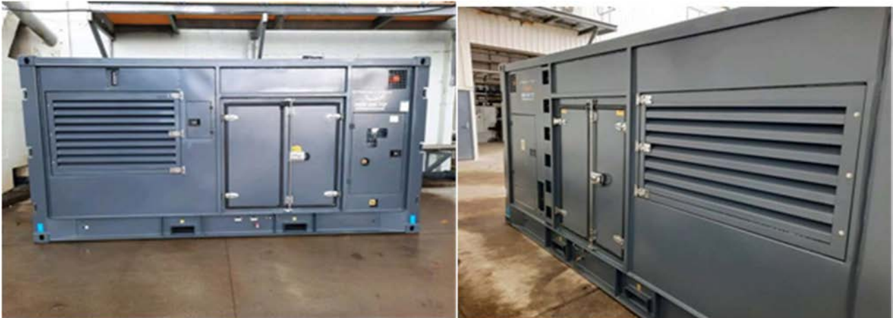
Kerepēhi Water Treatment Plant Containerised Generator
