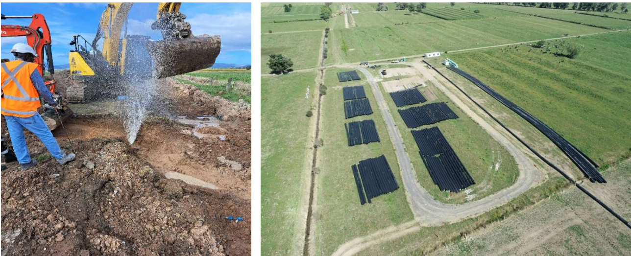
Picture to Left: Kerepēhi Raw Water Main – Undocumented Raw Water Connection. Picture to Right: 650mm Pipe from Pekapeka Intake to Kerepēhi Water Treatment Plant.
