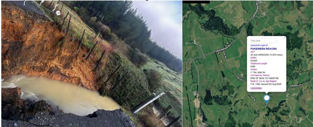
Image 3 & 4 – Pukewera road culvert washout & location
