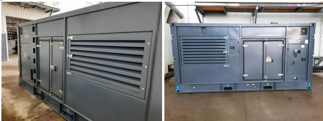
Kerepēhi water treatment plant containerised generator
