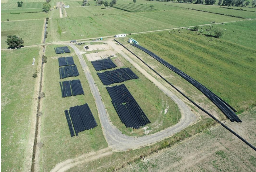
650mm-diameter pipe from the Pekapeka intake to the Kerepēhi water treatment plant.
