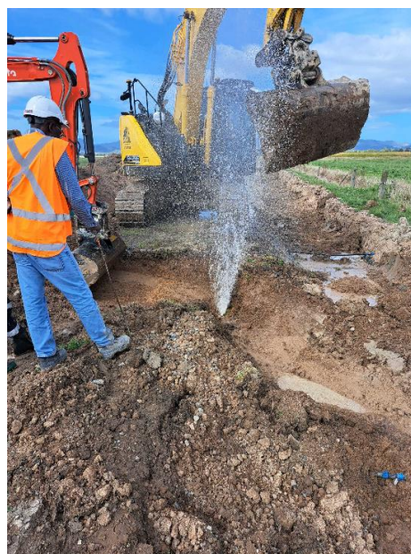
Kerepēhi Raw Water Main
