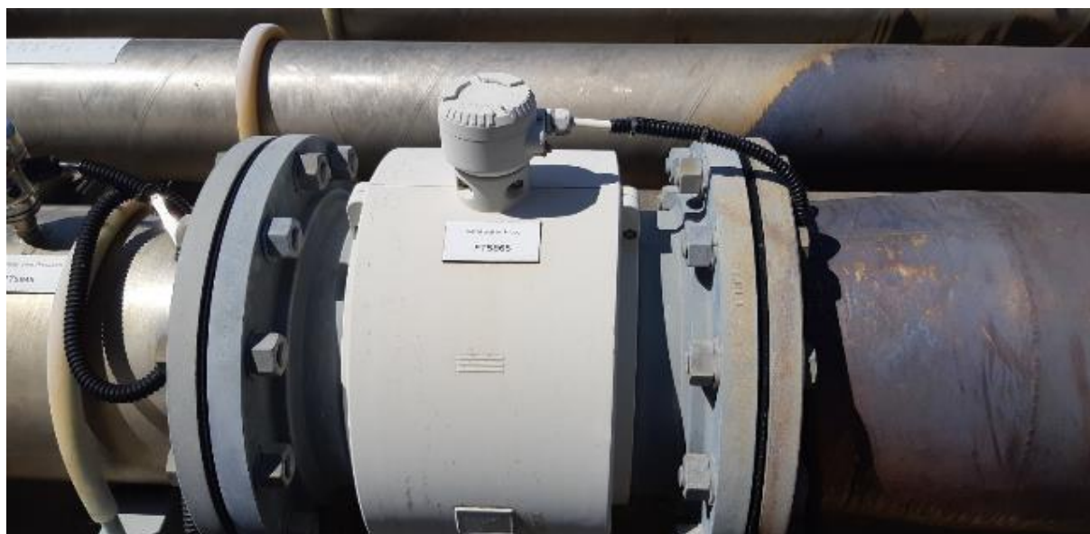
Figure 3: Dewatering totalising flow meter
