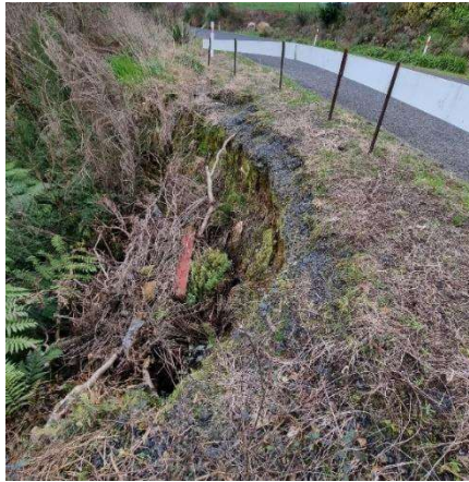
Figure 1 – Narrow & steep shoulder at Culvert 65, Chainage 0.66km
