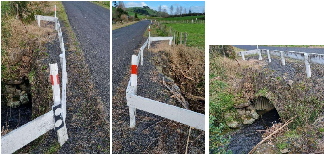
Figure 3 – Narrow & steep shoulders at Armco Culvert, Chainage 0.37km
