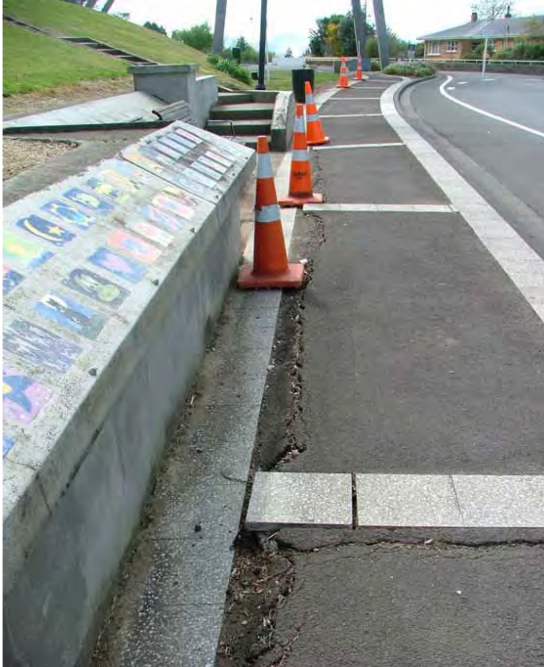
Photo 5. Ground cracking due to lateral northward movement and subsidence, evident along the base of the Millenium Wall in Seddon Street, Sept 2008.
