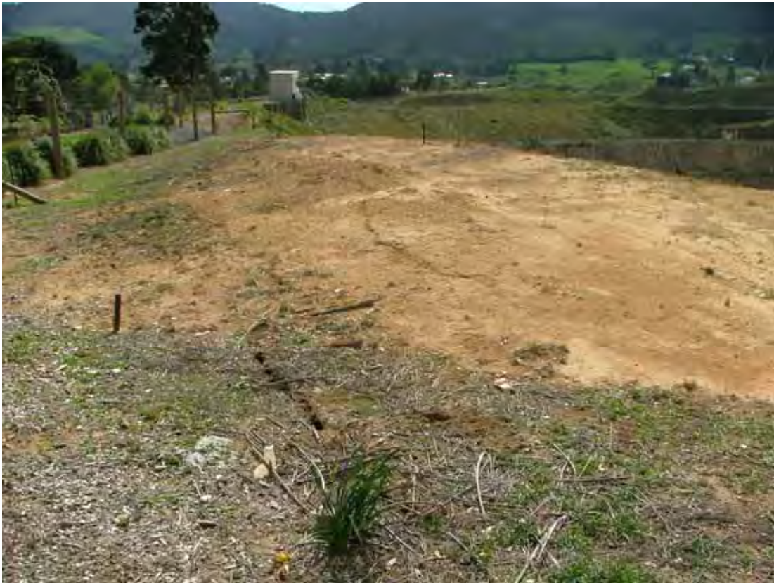
Photo 6 View of surface cracking near the open pit rim which is being monitored with wire extensometers. View looking west.
