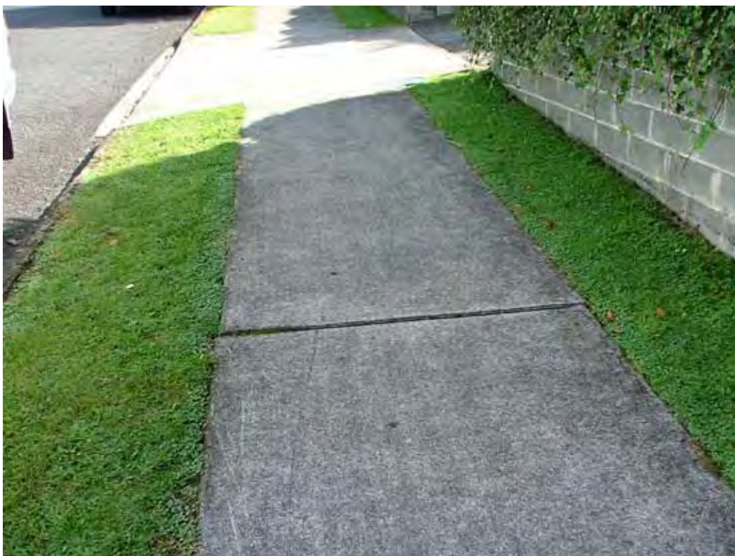
Photos 1&2 Cracking in Haszard Street with an unusual north (pit wall) side up and small right lateral component, suggestive of large “block” movement on a through-going rock mass defect.
