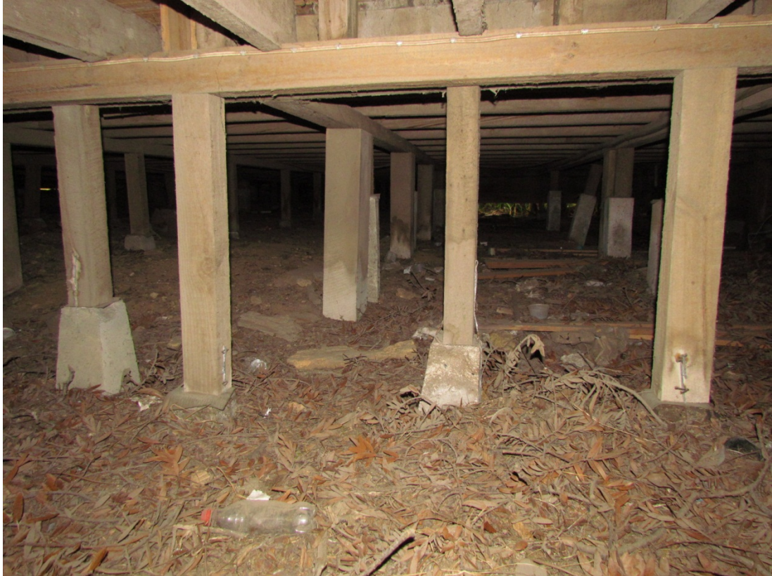
Sub Floor Framing – Note absence of sub-floor bracing
