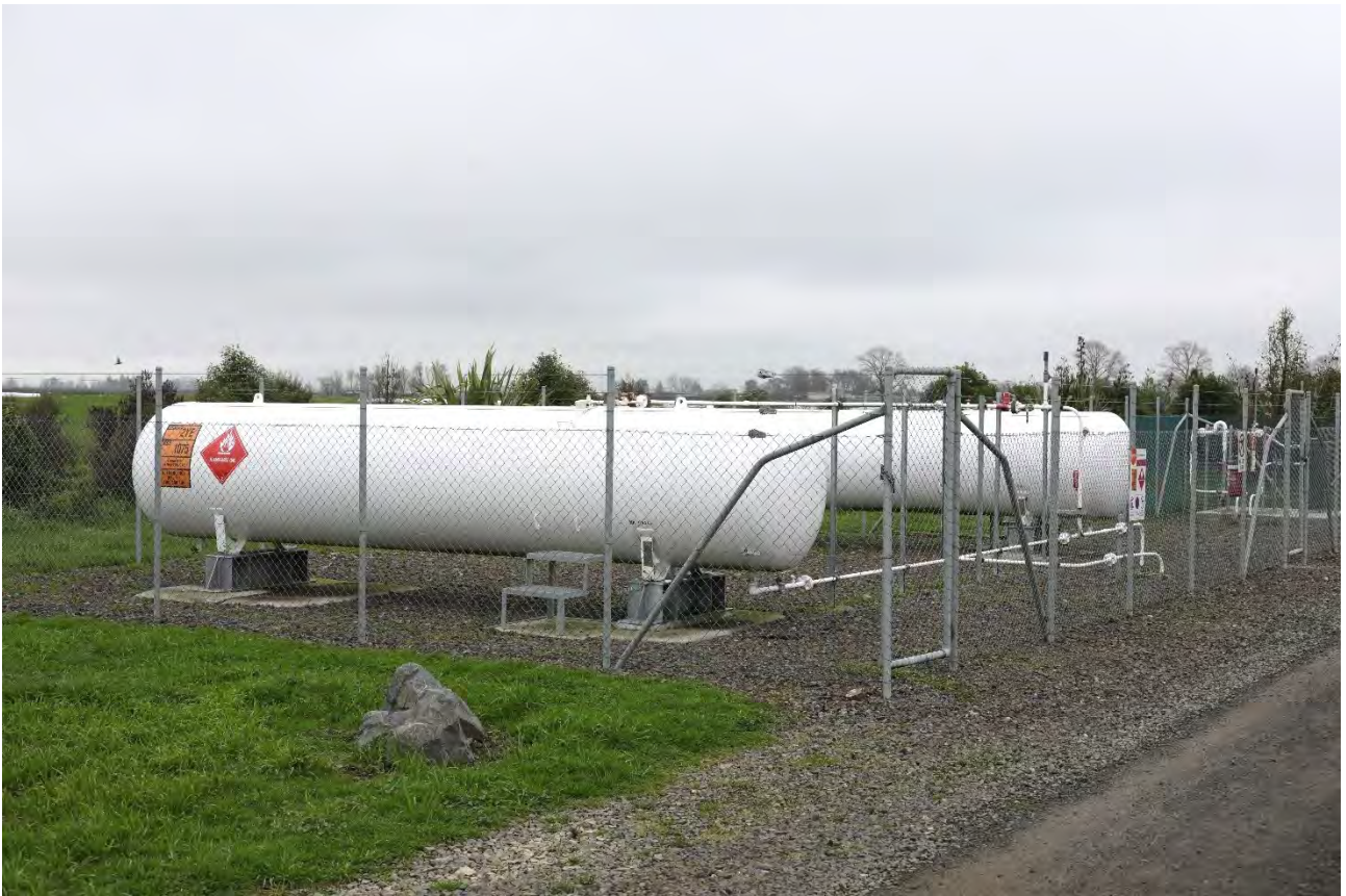
Figure 4: Wardville Broiler Farm example of LPG storage tanks and perimeter fence.
