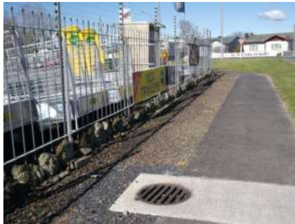
Figure 20: Catchpit at Ngatea Panelbeaters Ltd
