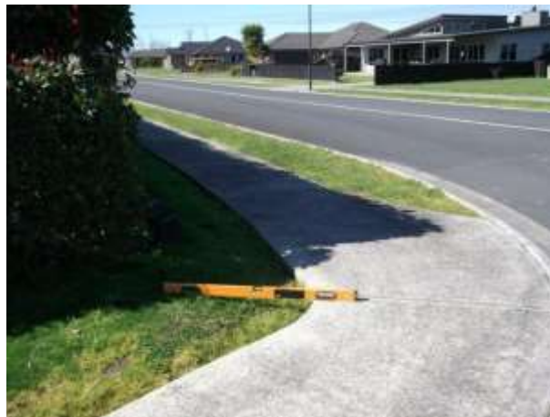
Figure 16: Low berm at 53 Darlington Street
