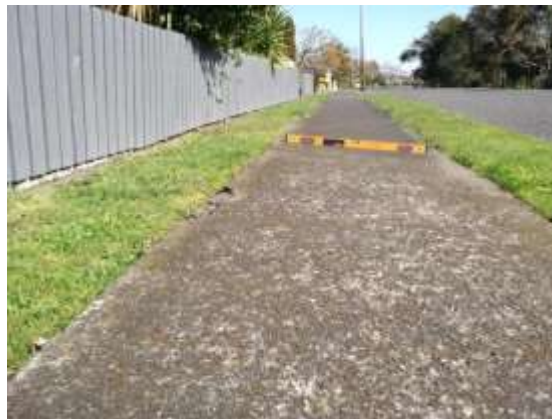
Figure 23: Crossfall of footpath at 37 Hayward Road
