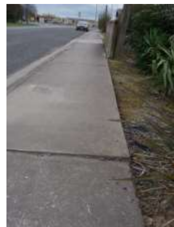
Figure 17: Lifting footpath on Kohunui Street
