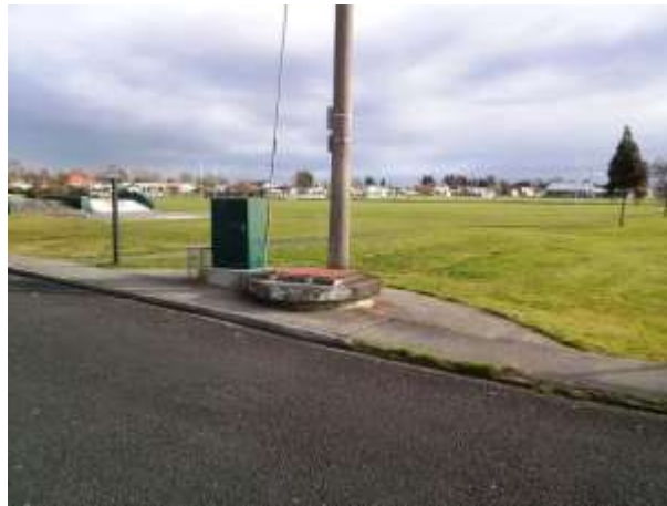
Figure 18: Service cover on Norwood Road
