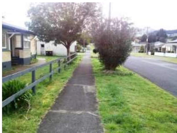
Figure 28: Broken footpath on Thorp Street at 168 Normanby Road
