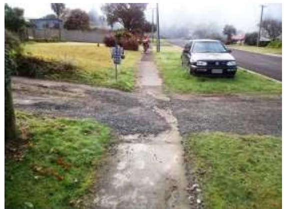
Figure 25: Loose metal from a driveway on George Street.
